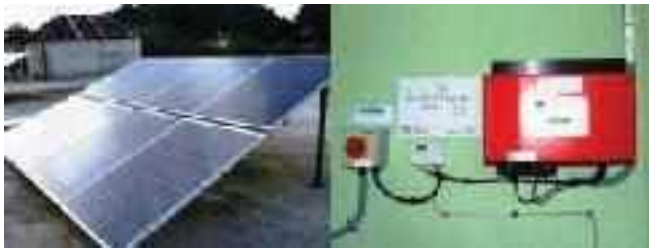
Solar panels of CRP-Savar
